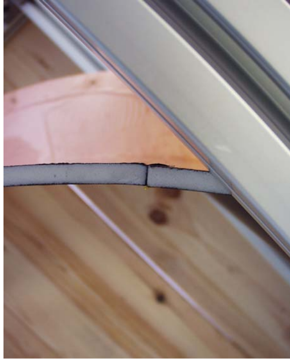
FIG 9 The Airex joint, showing some delamination.
