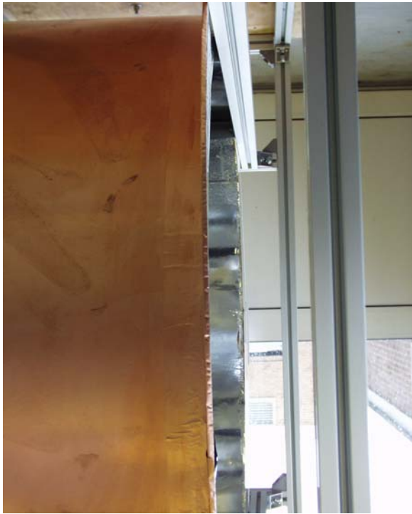
FIG 8 The Flange is not flat.
